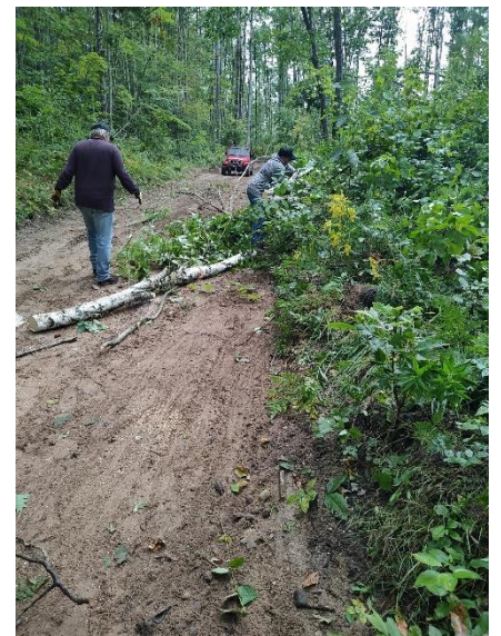
We had to cut trees into pieces to get to the chipper.
