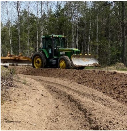
Russ worked the east side using the grader. Some high berms to knock down.
