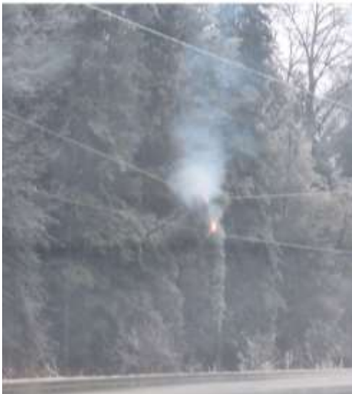
Power lines took major hits, catching on fire in some cases.
