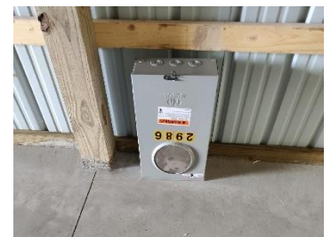
New electrical panel box ready to be installed.
